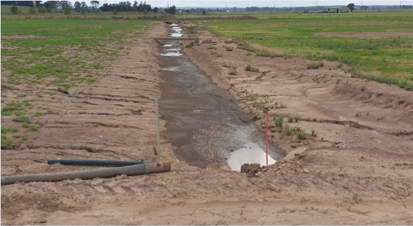
Bare earth drain
