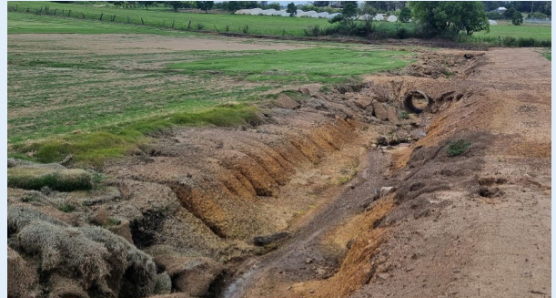
Eroded bare earth drain
